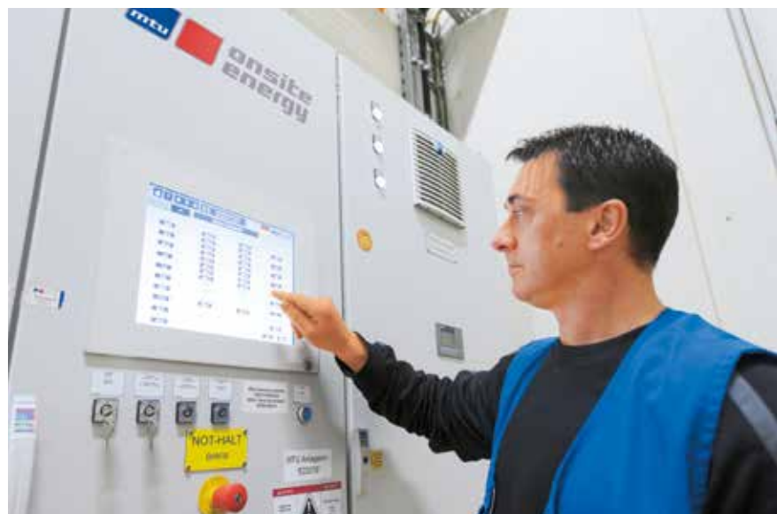
Two combined heat and power (CHP) plants from MTU Onsite Energy generate the power needed for brewing beer.
